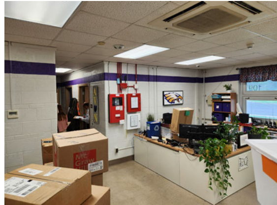
Fire Alarm Panel
