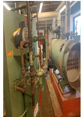
Hot Water Boilers
