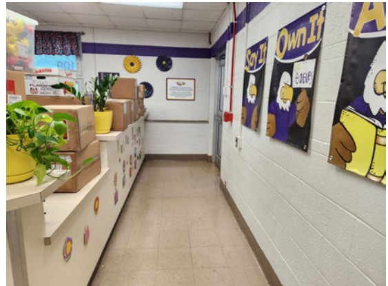
Fire Alarm in Office
