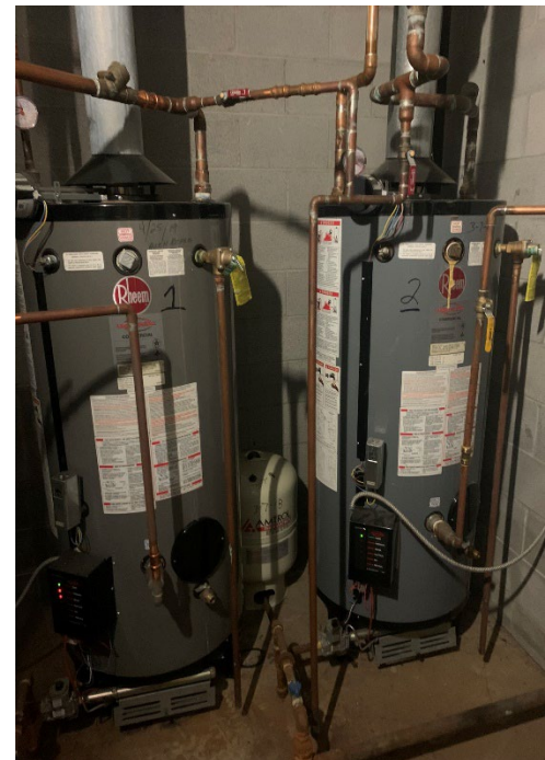
Gas-fired Domestic Water Heater
