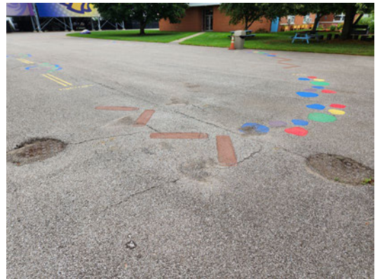
Cracked Playground Surface
