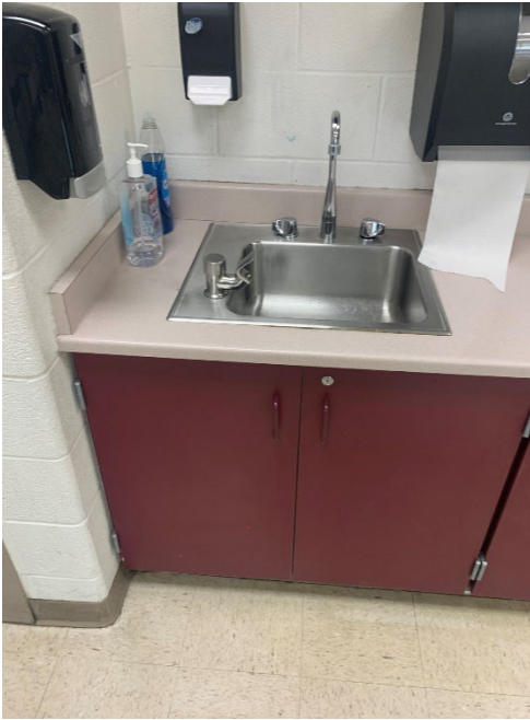
Classroom sink w/drinking fountain
