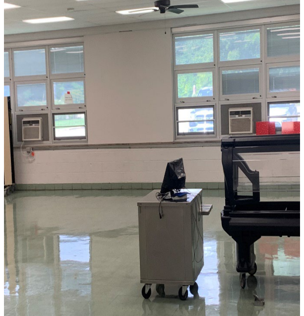
Window A/C Unit
