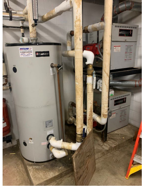
Gas fired domestic water heater and storage tank.
