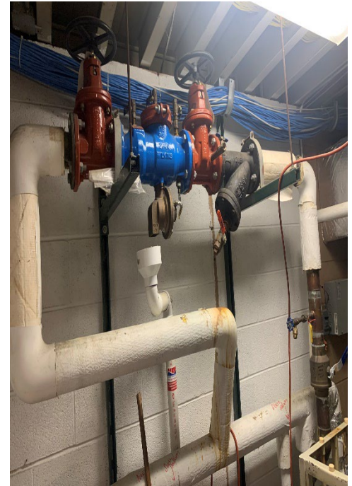
Water Service Backflow Preventer
