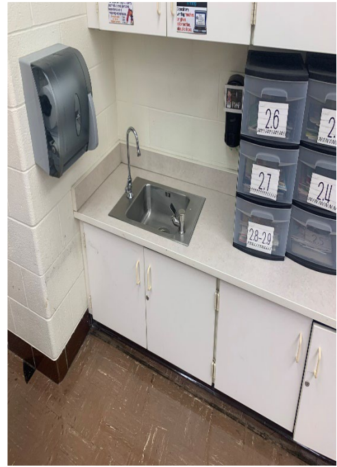
Classroom Sink with Water Fountain
