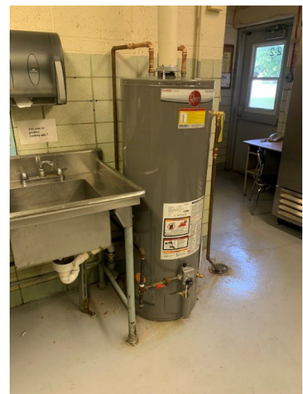
Kitchen Hot Water Heater
