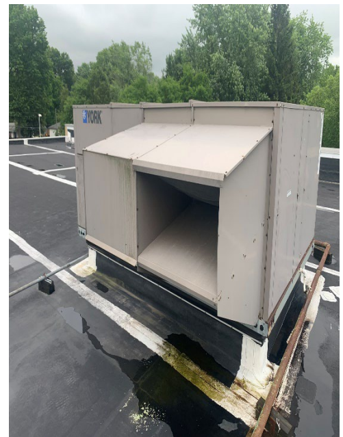
Single Zone RTU
