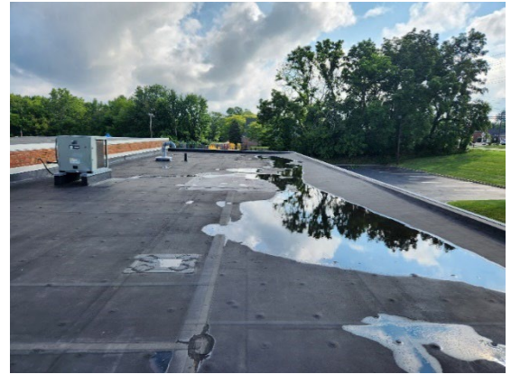
Standing water on Roof
